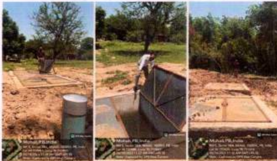
Photo 58: College's Rainwater Harvesting System
