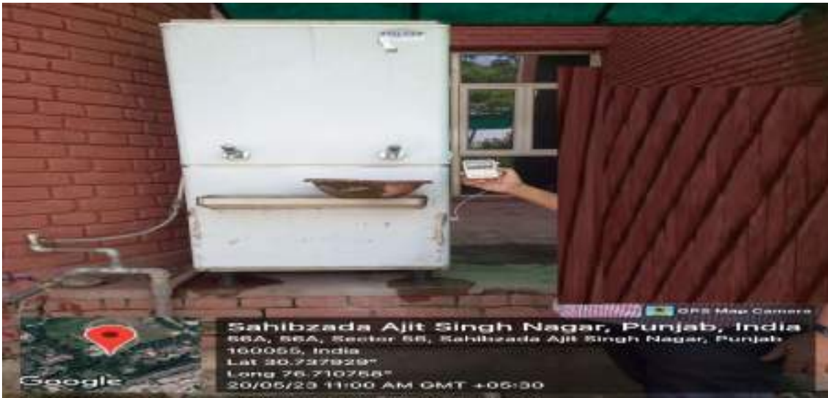
Water Cooler installed in the G. floor
