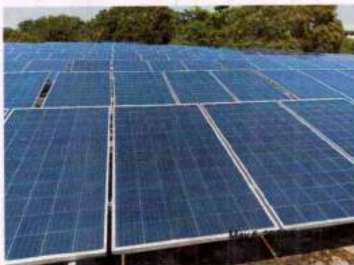
View of Installed Rooftop Solar Panels
