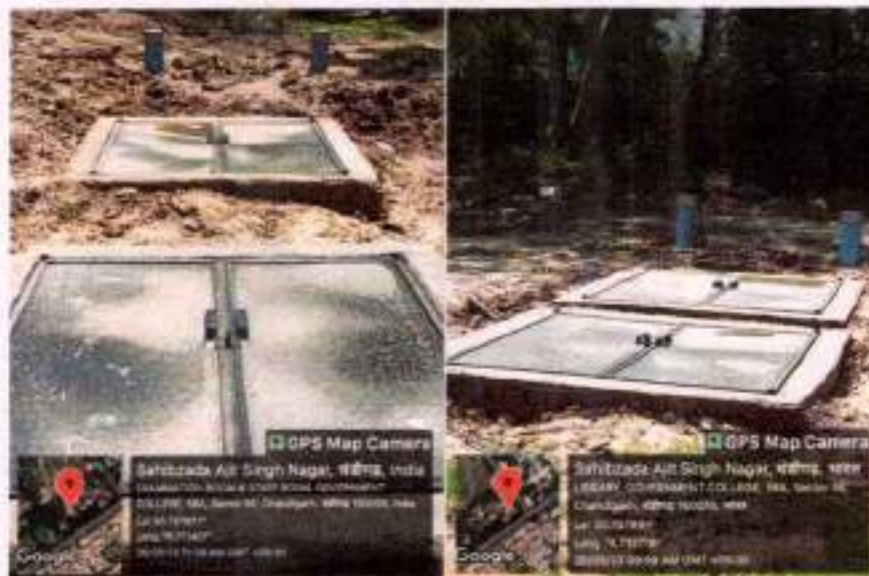
Photo 59: College's Rainwater Harvesting System
